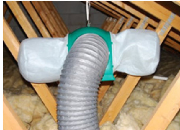
Figure 1 Roof located positive ventilation system
