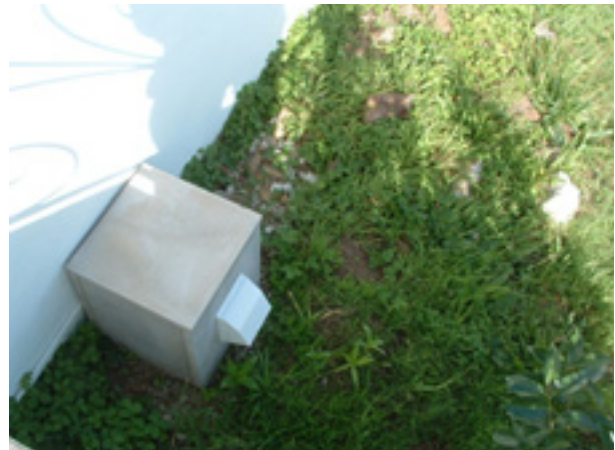
Figure 2 Fan located in a weatherproof housing made from concrete paving slabs
