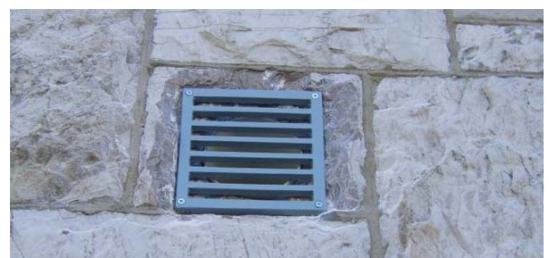
Figure 10: External air inlet vent to a wall-mounted positive ventilation system
