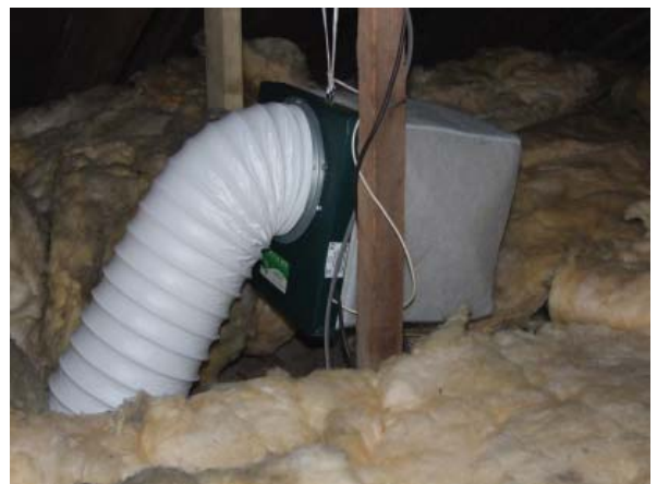
Figure 1: Roof-located positive ventilation system
