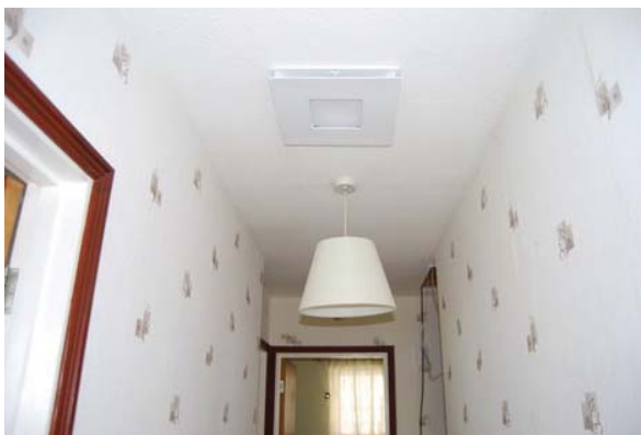
Figure 8: A ceiling diffuser located in a stairwell in a house or hallway in a bungalow
