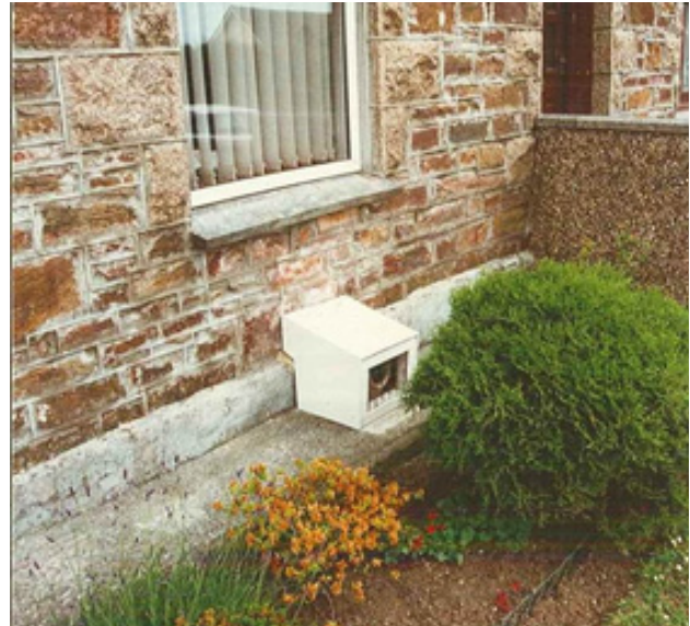
Figure 2 External fan in a weatherproof box
